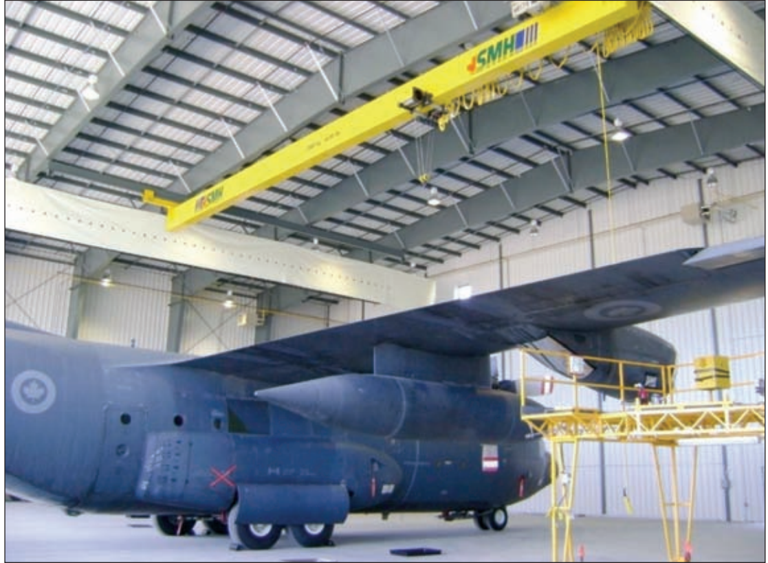
Figure B2: Under Hung Crane
