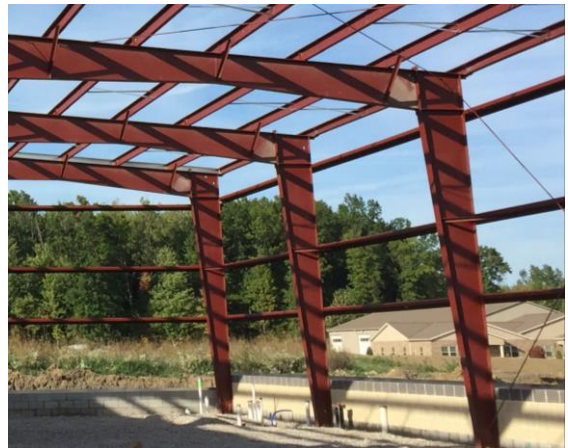
Girts and purlins attached to primary structural steel frames. Various types of bracing shown, such as x-bracing, flange bracing, girt and purlin bracing.
