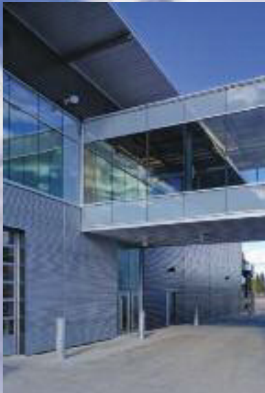
Bridge connecting Trade shops to the original Pine Ridge building, showing the unpainted AZM150 Galvalume 22mm (7/8") corrugated wall cladding.
