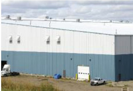
The building's steel standing seam roof is clad with 19,417m 2 (209,000 sq. ft.) of unpainted 61mm (.0239") AZM165 Galvalume Plus, with an acrylic coating.
