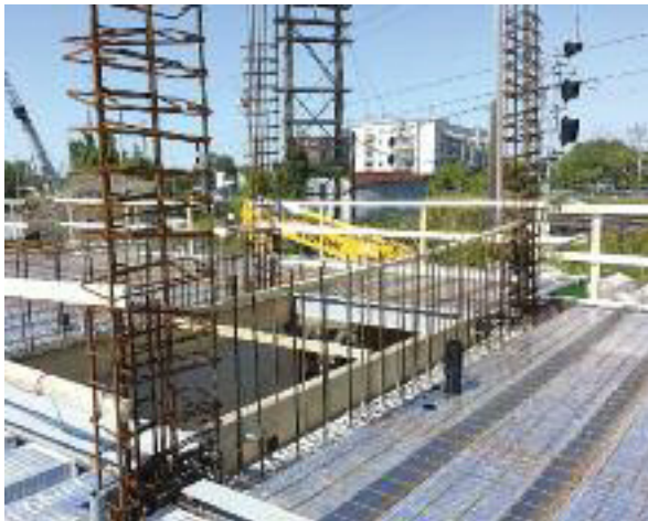
Axcès Saint-Charles in Longueuil, Québec, built with the UltraBond composite floor system and light steel framing. Rebar creates reinforced beams in the UltraBond composite floors, using 22mm (.048") Z275 (G90) galvanized steel.
