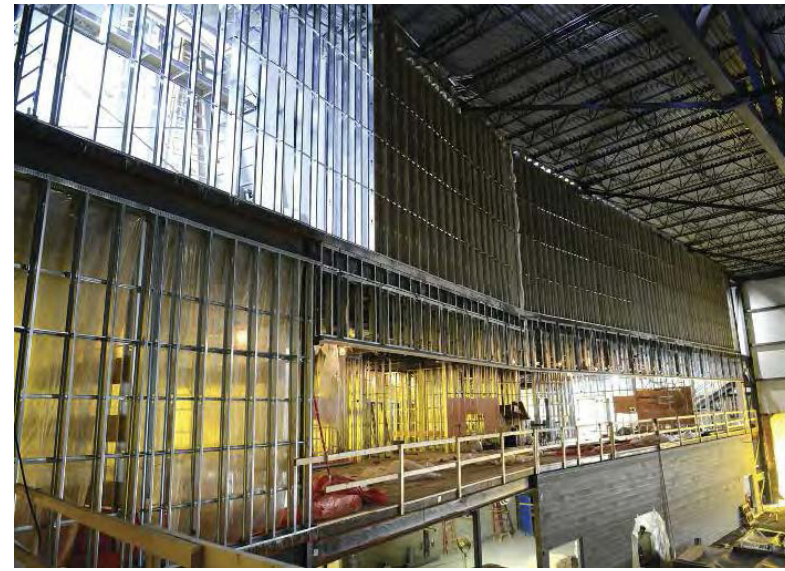
Interior arena, west facing – extensive use of cold formed sections for exterior walls.
