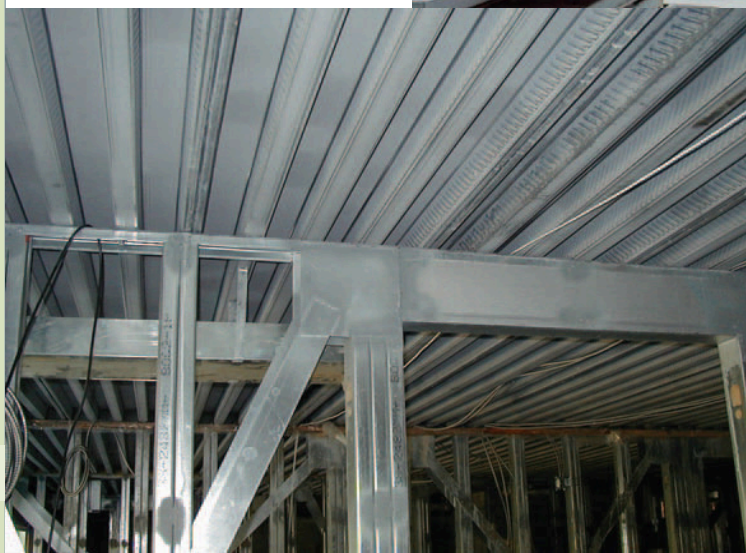
Intersection of the walls and floor system. The deck is 75 mm (3") x 1.22 mm (0.048") composite deck by Vicwest, and the studs are 90 mm (3-5/8") x 1.52 mm (0.060") studs.
