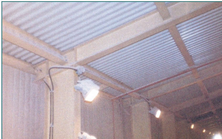
Figure 7: Potash plant, raw ore storage interior. A hot and humid potash environment containing potash dust. Note potash build-up on light fixtures. Eleven years exposure in Saskatchewan.
