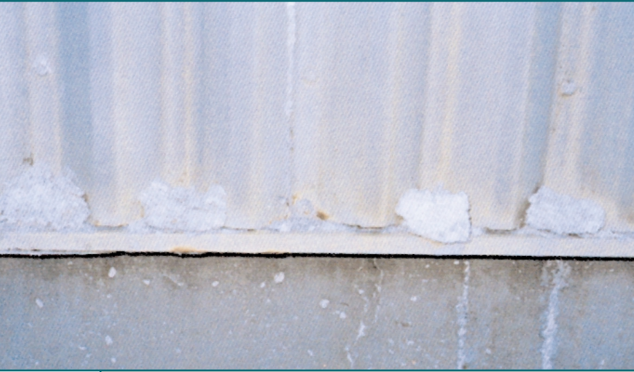
Figure 4: Pulp & paper plant, recovery boiler building. Ground level west exposure below exhaust duct showing contaminate build-up and minor edge creep on the cladding. Eleven years exposure in Northern Ontario.
