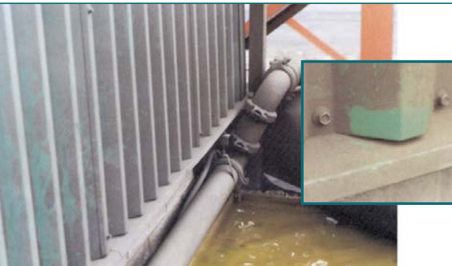
Figure 1: Mine water cooling tower. West exposure above the tanks. Insert: A quick cleaning showed that the drip edge was in excellent condition. Eleven years exposure in Northern Ontario.
