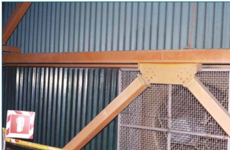
Figure 3: Mine refinery building interior. The Barrier Series cladding is above the exhaust fan. Eleven years of exposure in Northern Ontario.
