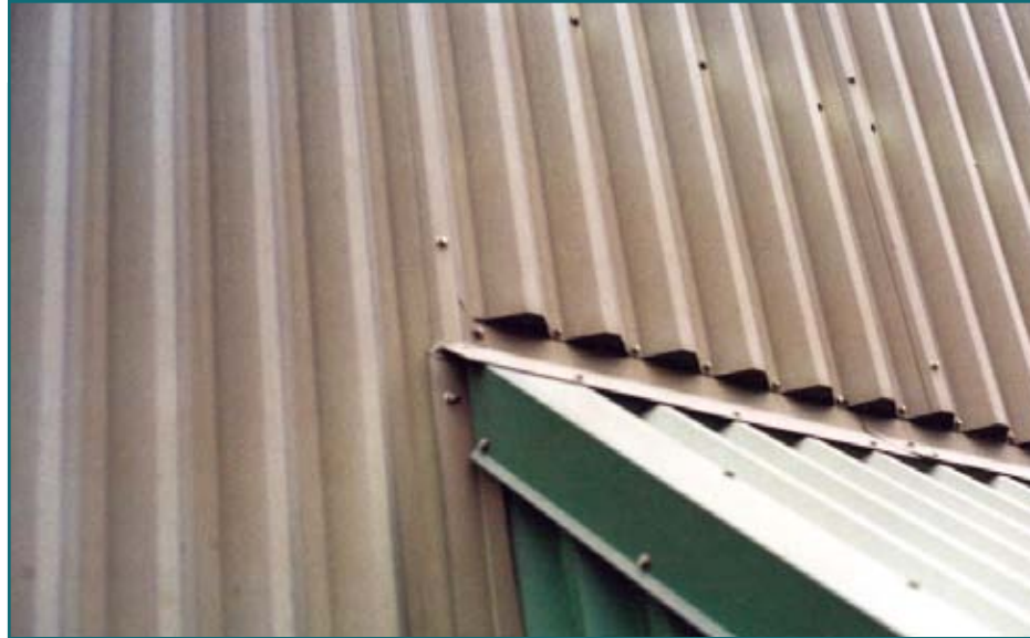
Figure 2: Mine smelter building exterior. Base edge and 45° angled cladding exposure. Nineteen years exposure in Northern Ontario.
