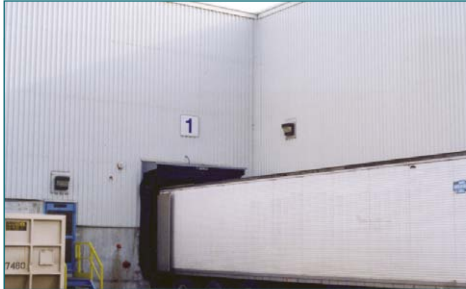
Figure 6: Kraft fine paper plant, paper finishing building. Comparison of new and old nine-year cladding. The newer cladding is on the right. Location in Northern Quebec.
