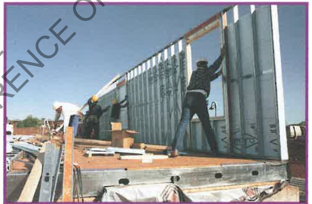
Four framers lift and hold a 40 foot lightgauge steel framed wall during construction of the Oakville Homesteel Project.
