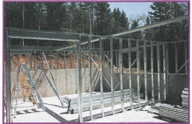
Loadbearing steel framing used in the basement of the Bedford Homesteel Project.
